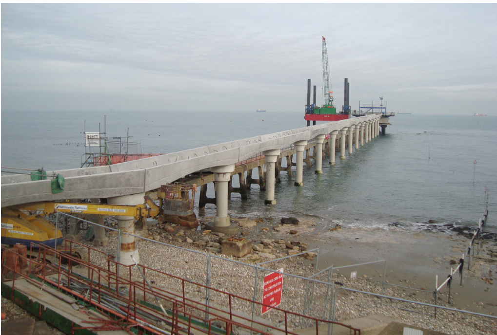
Work in progress! Bembridge Lifeboat Station – walkway to Offshore Boathouse (Photo by Paul Rainford)
